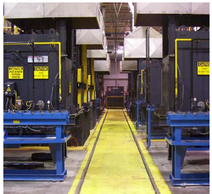
Bodycote’s heating plant uses Honeywell wireless technology to obtain needed information to monitor gas consumption
