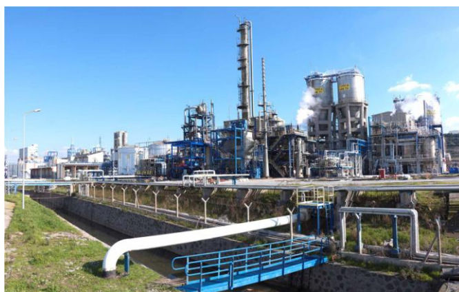
Petkim Petrochemical's flagship ethylene unit uses Honeywell's Profit ® Suite to maximize feed rate and minimize energy consumption.
