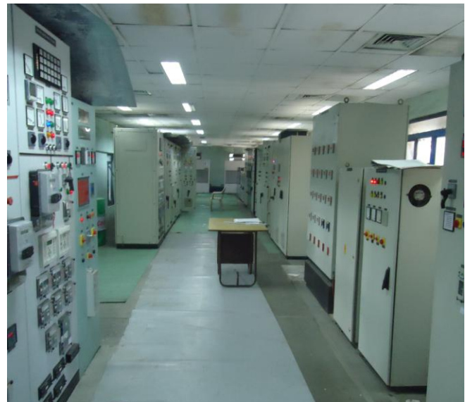
The Control Room at Sri Prabhulingshwar Sugars and Chemicals Ltd
