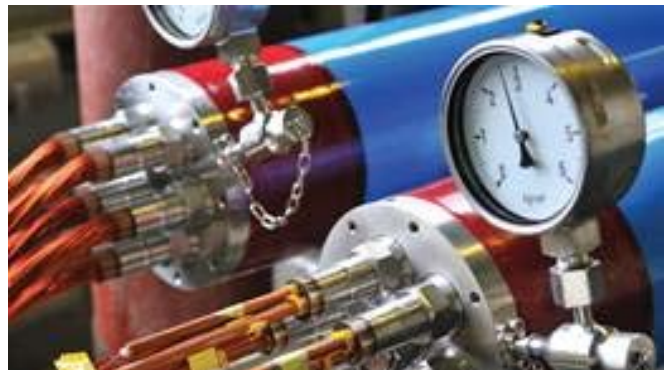
Honeywell HC900 controller replaced obsolete technology, reducing wasted power and providing additional process security.
