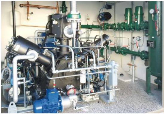
4-stage CNG Compressor Type 4DA 300 with Upstream Natural Gas Treatment
