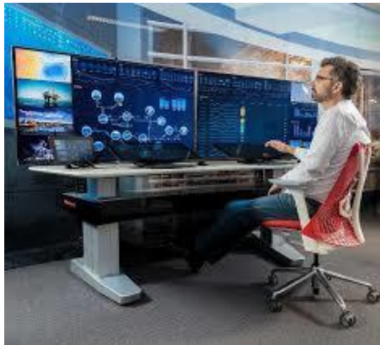
Figure 4: Industrial organizations upgrading to the latest automation technology will enjoy improved operational efficiency, greater process reliability, and increased plant productivity.
