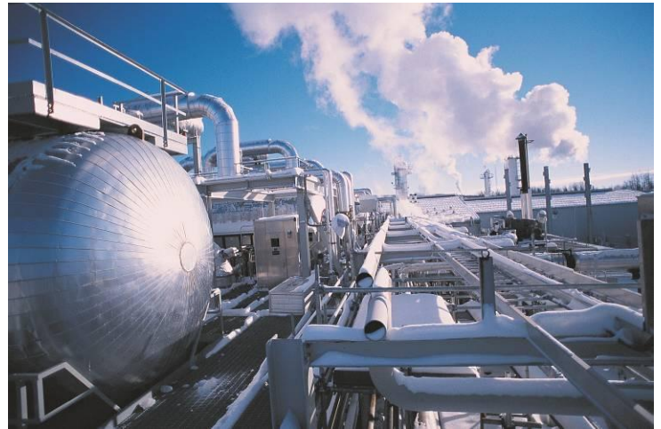
Fig. 1. For process plants, best practice operation means ensuring maximum yield, utmost efficiency and minimum emissions
